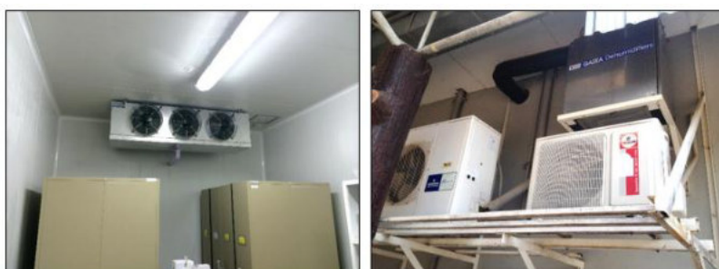
Figure 8 Refrigeration and Dehumidify system of Seed lab
