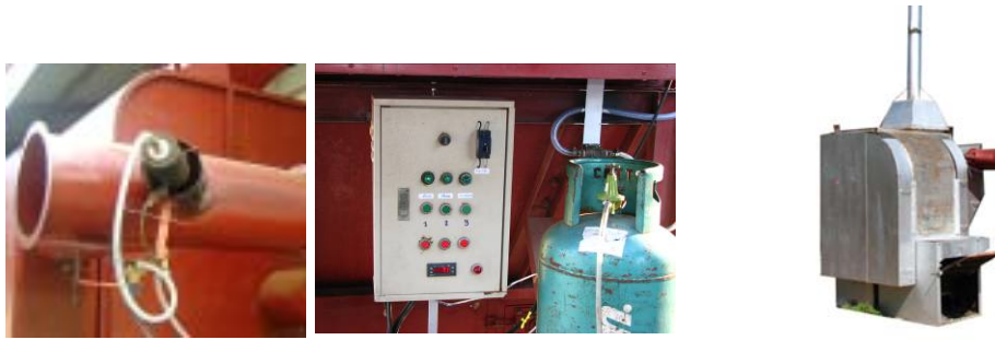
Figure 13. Gas burner together with temperature controller and heat exchanger of biomass furnace
